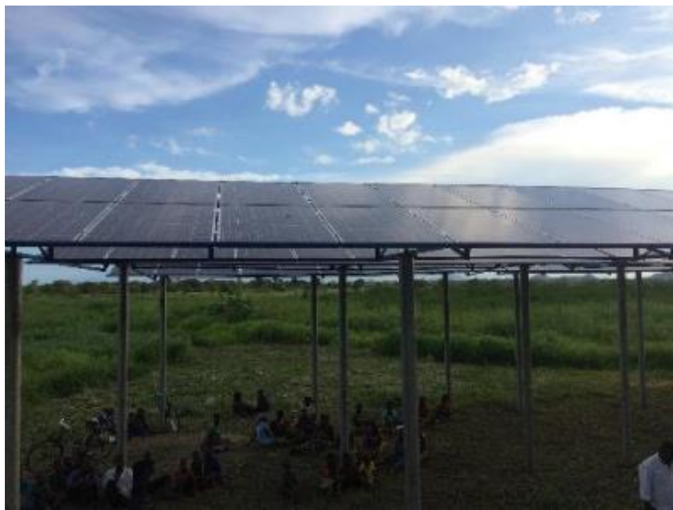
Solar panels providing energy to the FISD irrigation scheme
