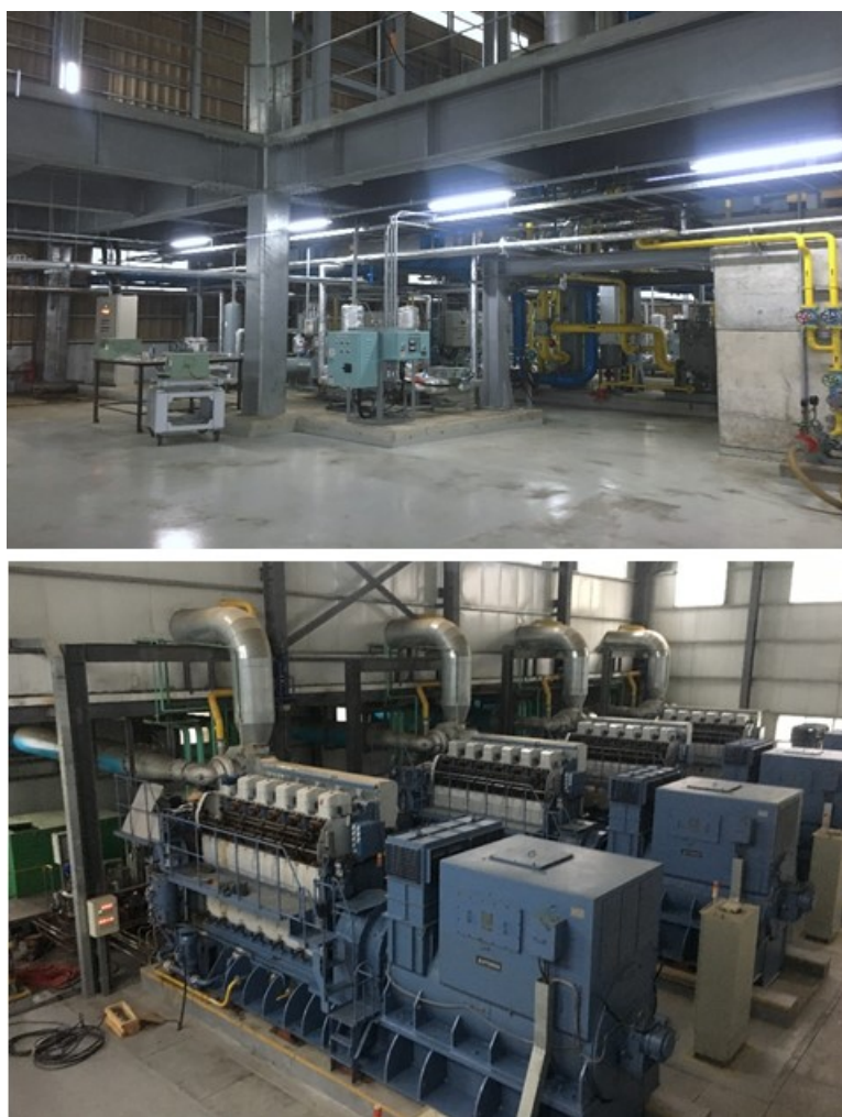
Figure VII.I. Bushrod Power Plant
