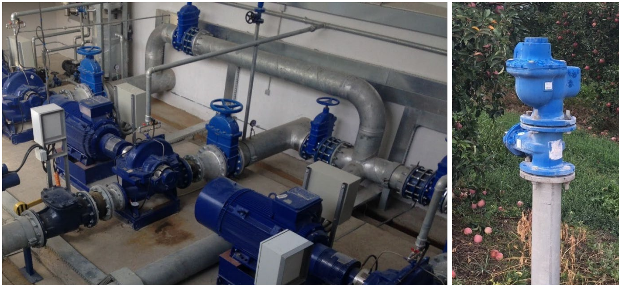
Figure I.2. Centralized irrigation system infrastructure
