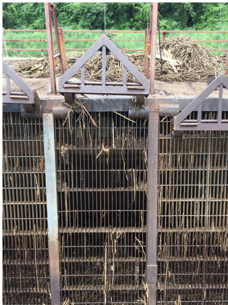
Figure IV.1. Intake screen with weeds (Nkula power station)
