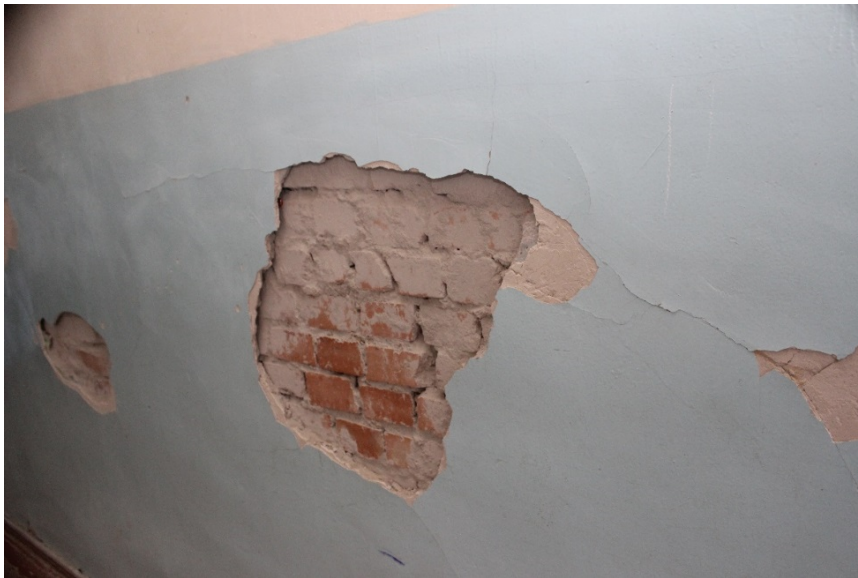
Figure IV.1. Illustration of damage in classroom walls
