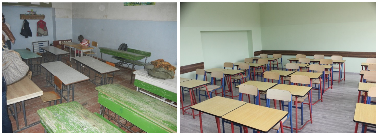
Classroom in need of rehabilitation
