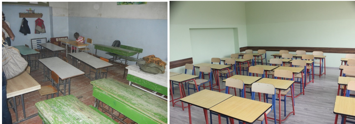
Classroom in need of rehabilitation
