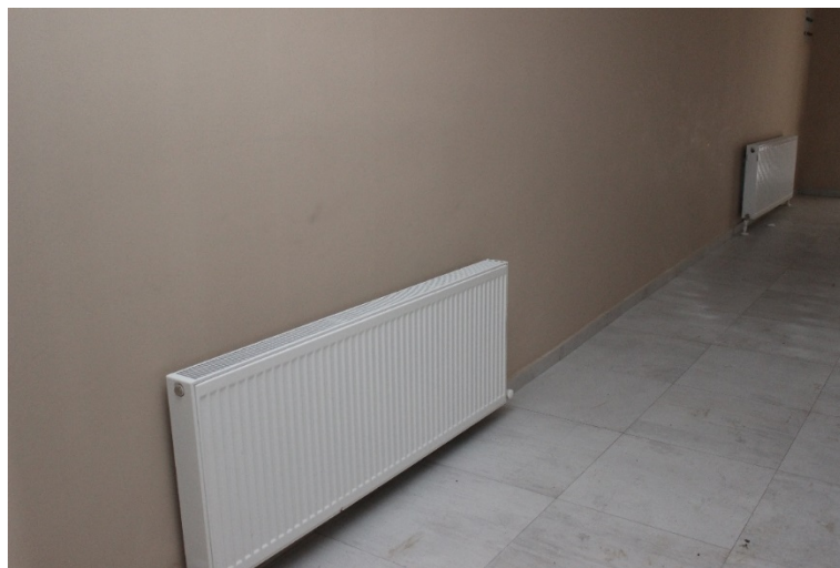
Central heating in rehabilitated classroom
