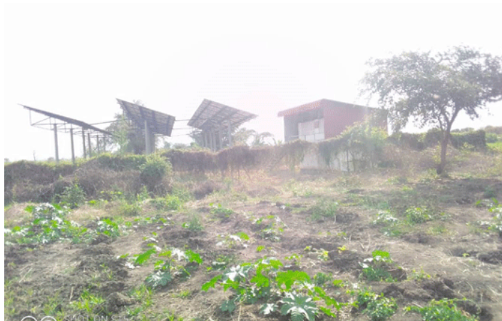
Photo: Water pump house and solar panels
