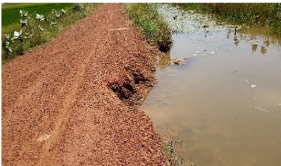
Eroded and flooded access route
