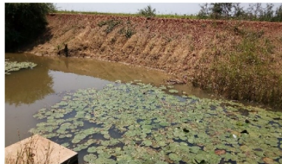
Eroded protection levee
