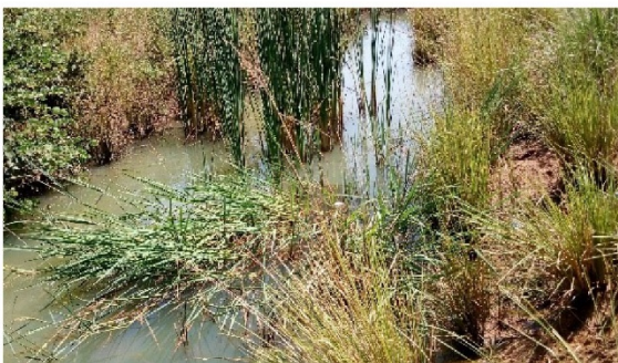
Clogged primary drain
