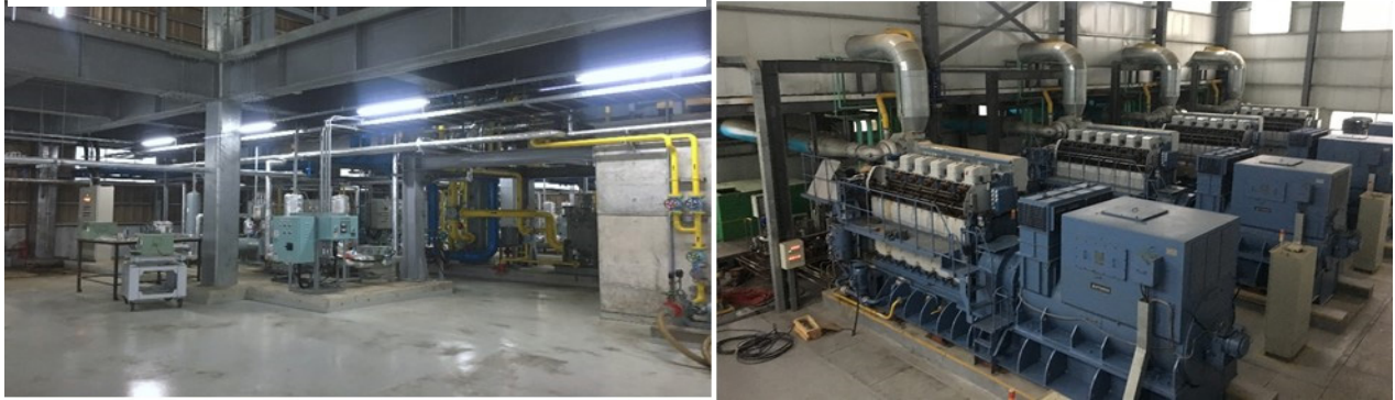
Figure V.8. Bushrod Power Plant, thermal generators
